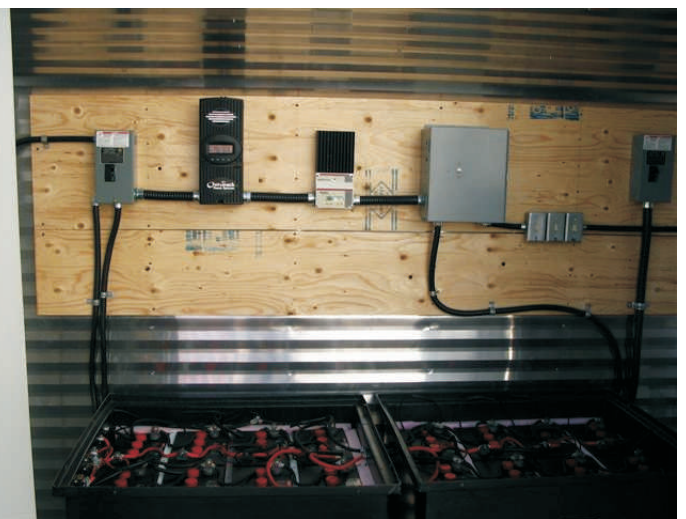
Batteries and controls
