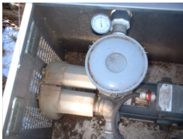
Solar powered air pump
