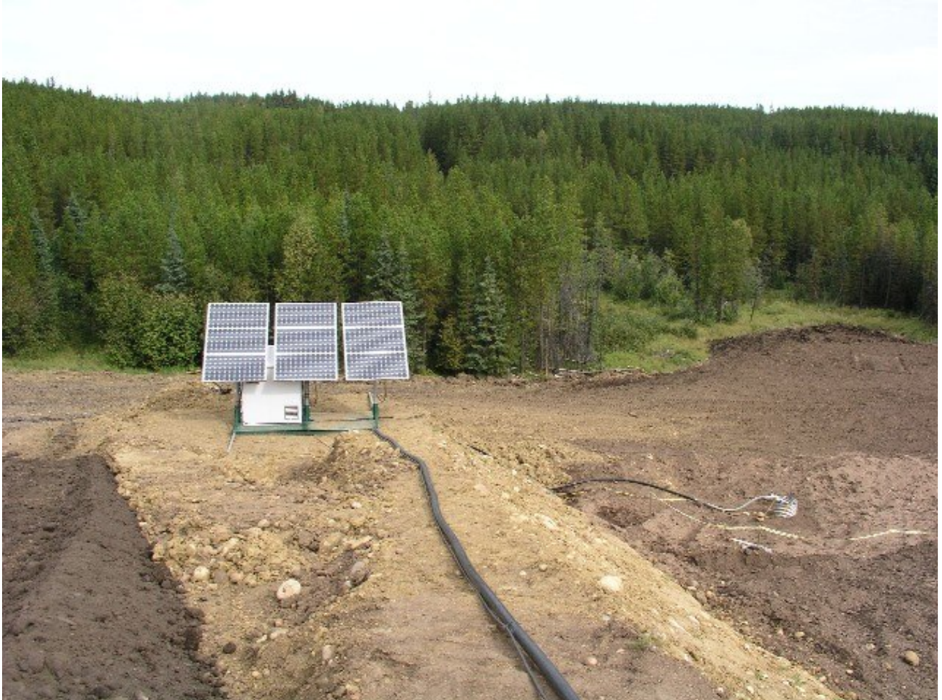
Solar pumping skid for Birchill Energy - Fox Creek
